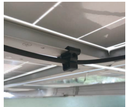
Outside the frame, wiring in parallel.
