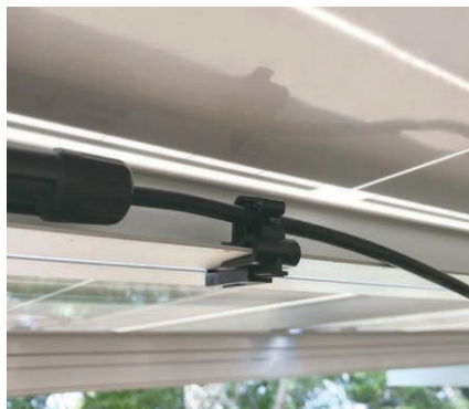
Inside the frame, wiring in parallel.
