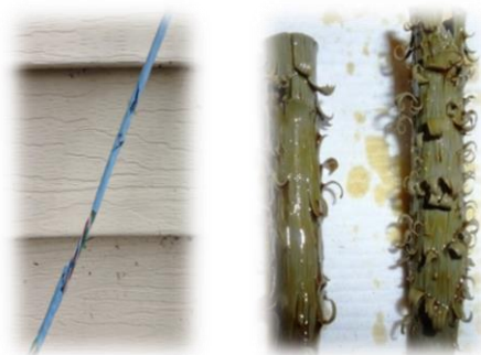
Figure 8. UV/temperature damage (left) and oil damage (right).*
